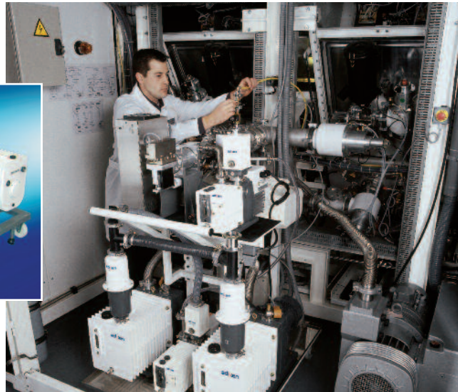
Pumping unit integrated in an industrial Leak Detection System
